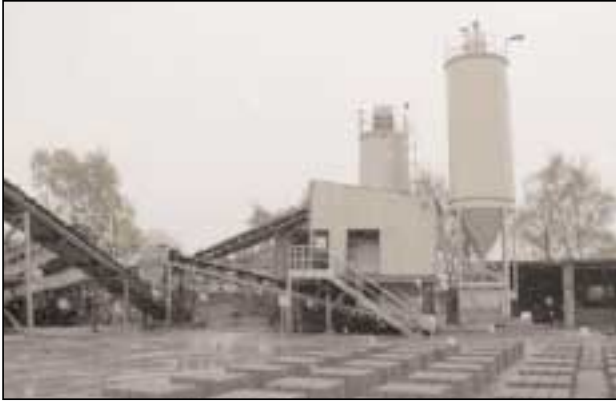
Figure 6. Block manufacture with FBA using 'egg laying' technique (courtesy of Innogy plc)
