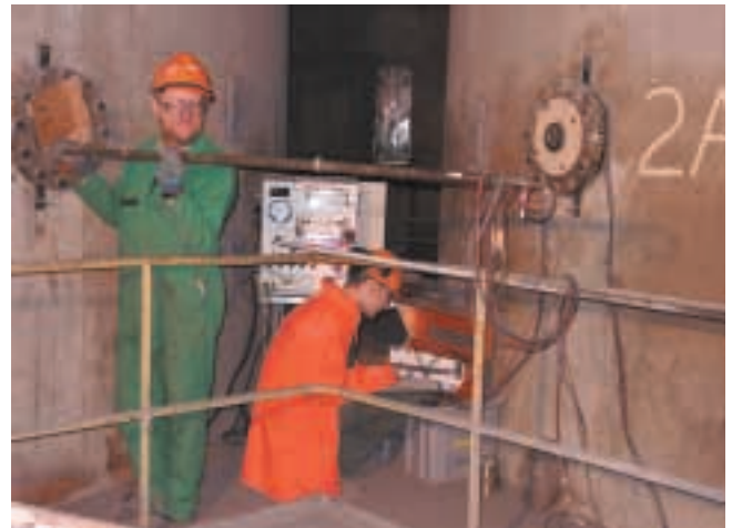
Figure 5. Flue gas sampling in-stack (courtesy of Powergen)
