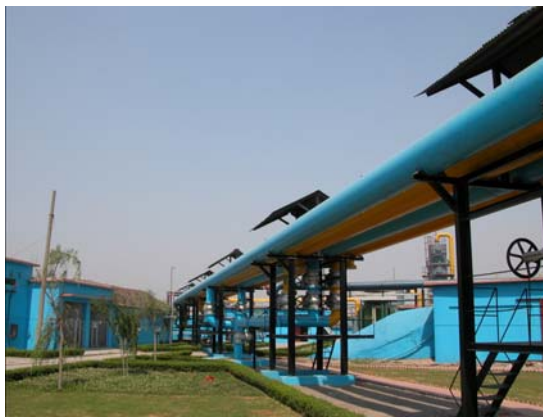
Erzhuang UCG Station – Xinwen Mining, Laiwu, Henan Province, China (courtesy of Xinwen Mining)
